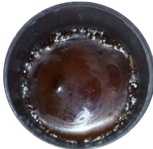
Fig. 2. External view of the cable inlet back surface with a flat penetration defect (0.1 mm thick, 4 mm high, 57 mm long)
